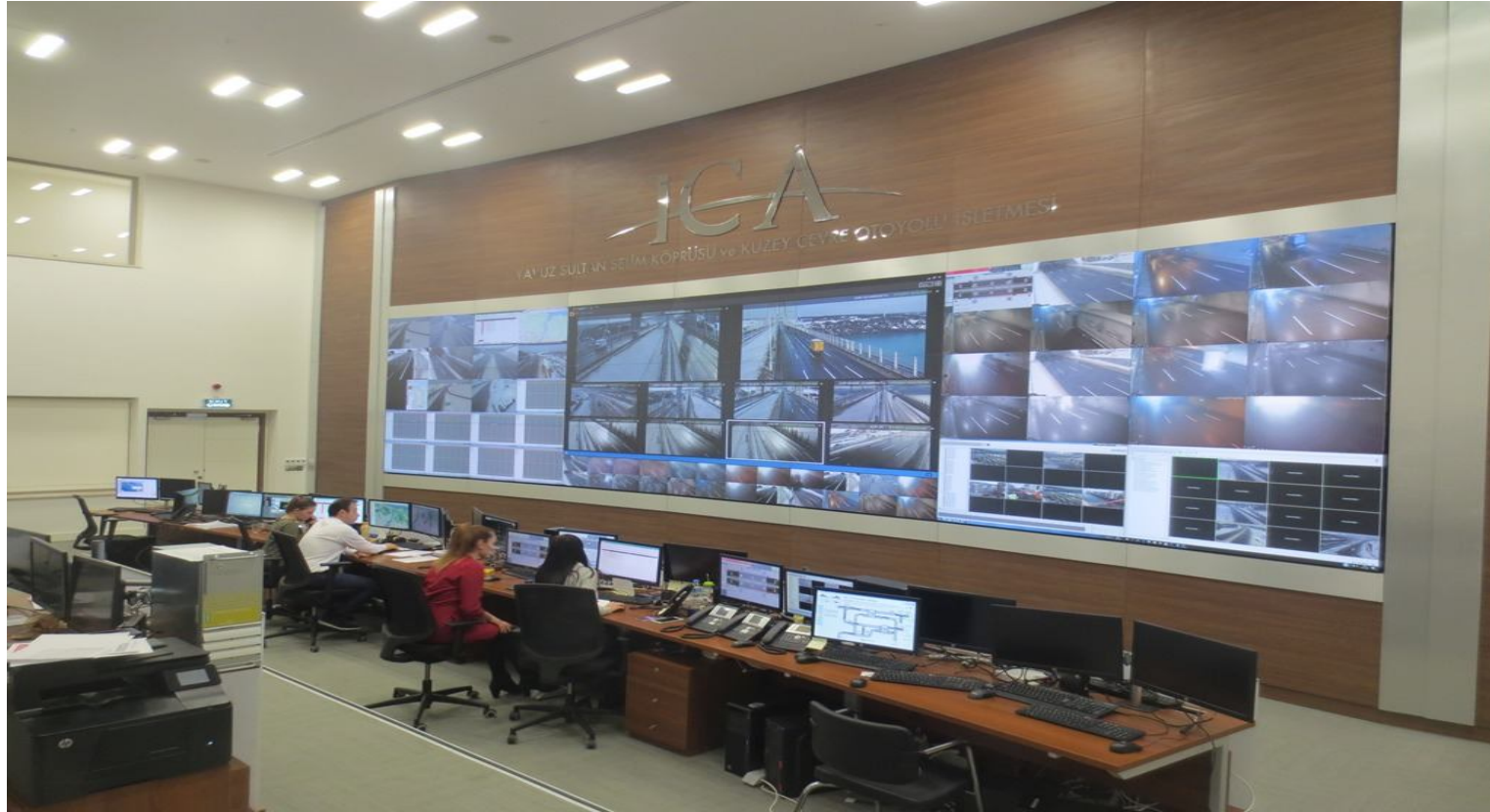
Yavuz Sultan Selim Bridge Main Control Room
