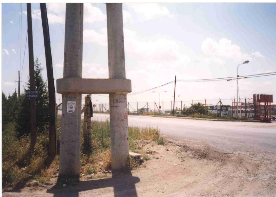
Example of dangerous obstacle close to the road.
