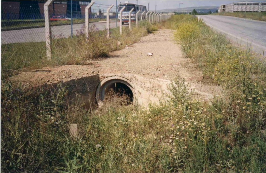
Example of dangerous culvert ending close to the road.
