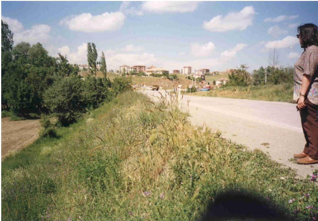
Example of a high and steep side slope without guardrails.
