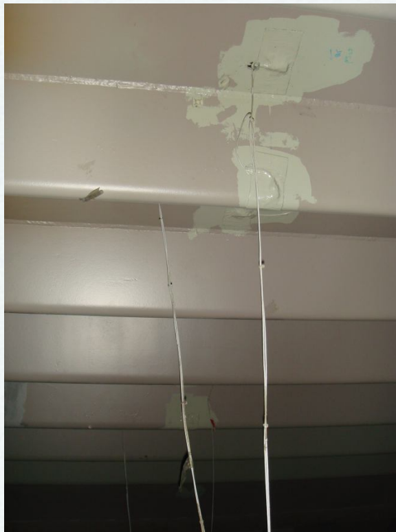
Strain gauges in deck
