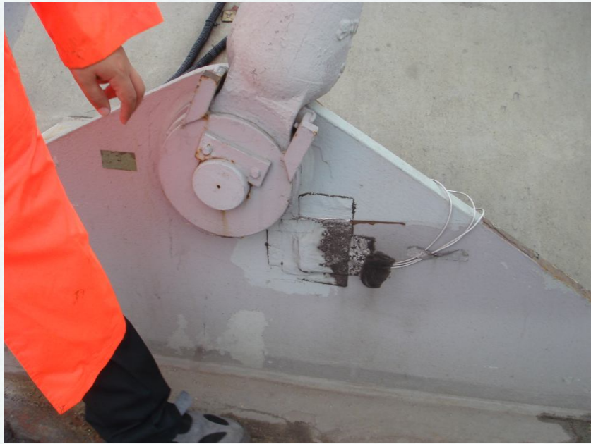
Strain gauges on hanger plates
