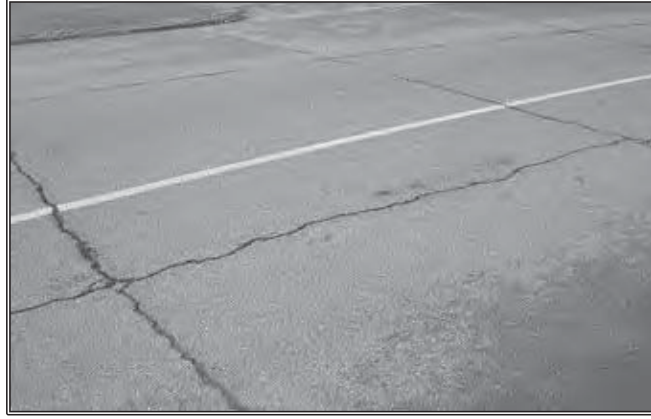
řekil 3.6. Yansima atlalı (Reflection Cracking)
