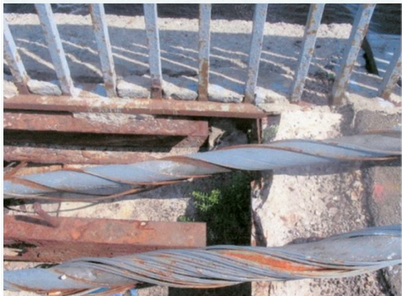
Defects of cables
